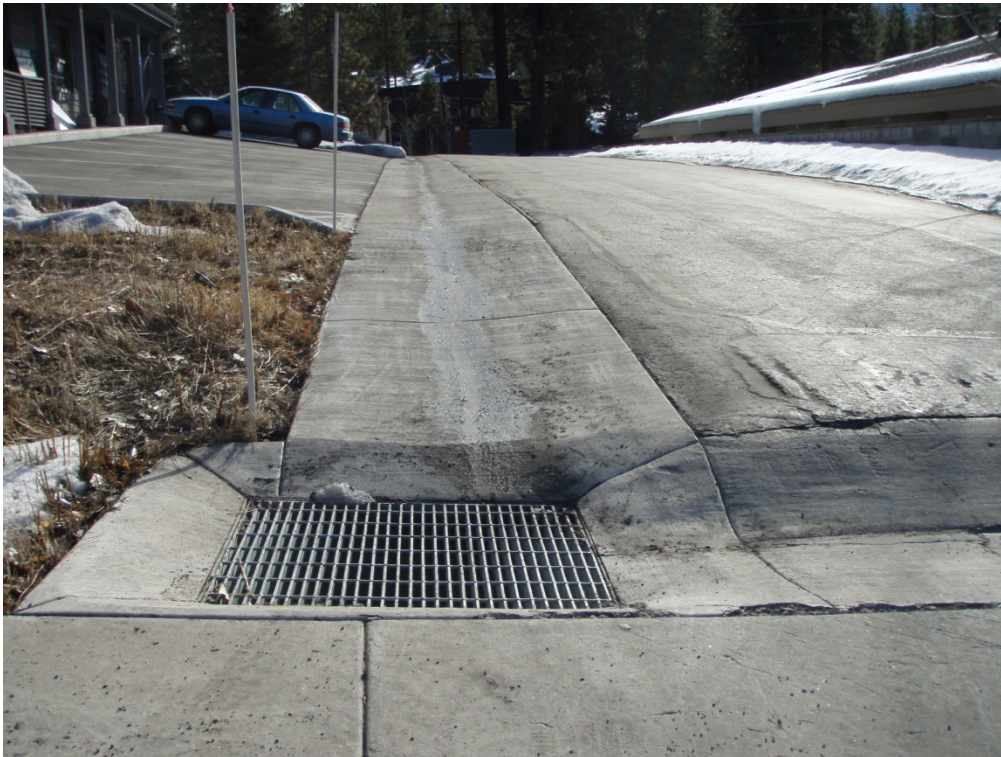
A drop inlet collects stormwater from a parking lot.
