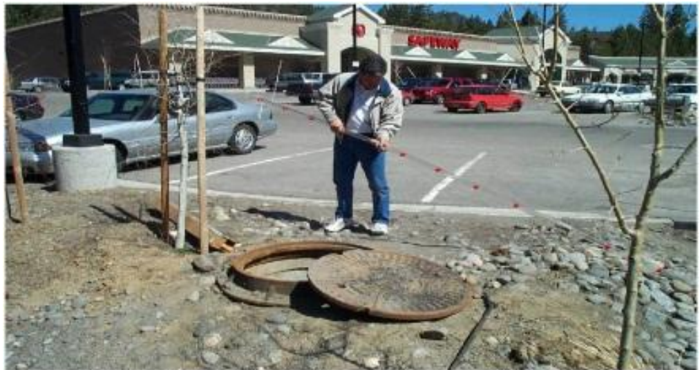
Inspection of a baffle vault to determine the depth of sediment accumulation and whether oil/grease absorbent pads need replacement.
