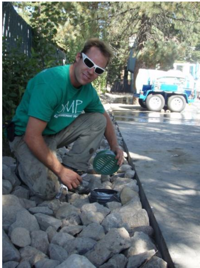
Contractor showing an inspection port open to visually assess for sediment accumulation in a rock infiltration trench.
