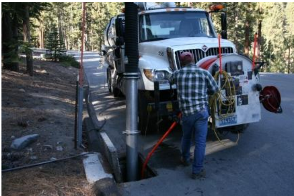
Vactor equipment removes sediment and other debris out of a drop inlet, preventing re-suspension of materials into the storm drain during the next storm event.
